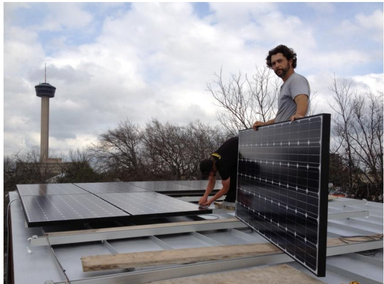
Installation of the 6 kW PV system. The system is completely hidden from view from the right-of-way. This allowed the project to comply with historic designation regulations and ensured optimal exposure for the panels.
