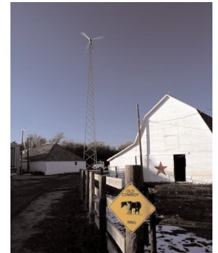
Bergey WindPower 10kW XLS turbine
