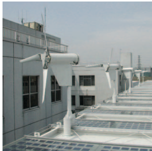
Proven Energy 2.5kW turbine rooftop array
