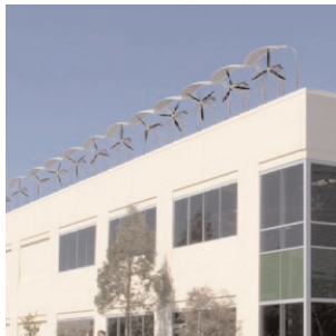
AeroVironment rooftop array
