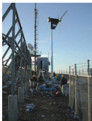
Proven Energy 6kW turbine powering telecommunications equipment
