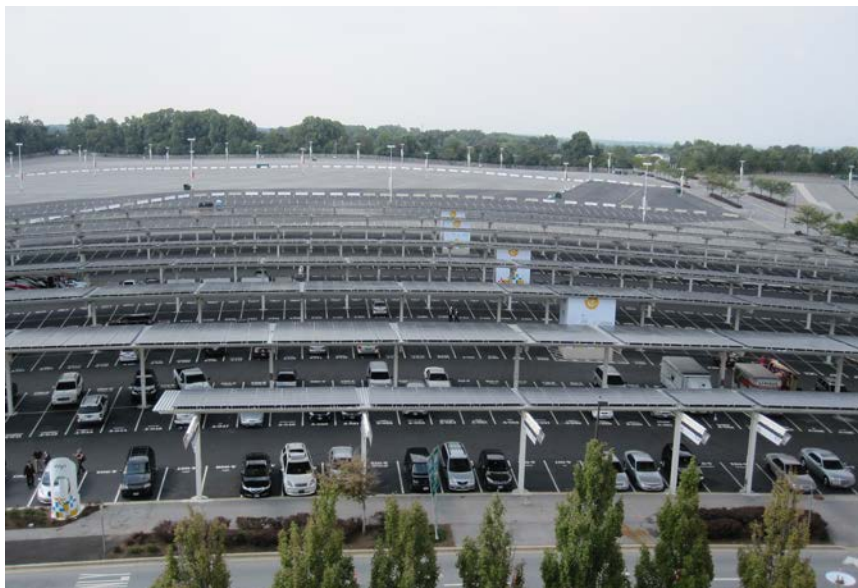
Solar Panels at FedEx Field.
