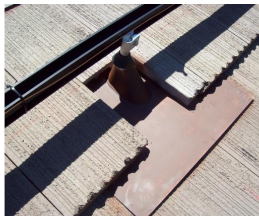
Figure 15 properly installed flashed roof penetration (correct)
