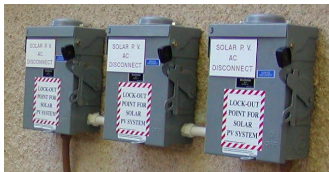
Figure 21 sign in PV ac disconnect (correct)
