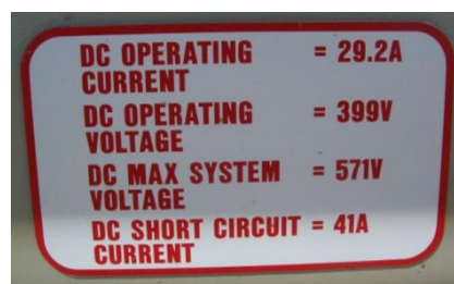
Figure 20 PV Power Source sign (correct)
