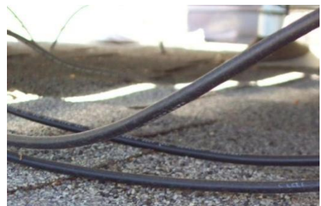
Figure 3 USE-2 conductors touching roof surface
