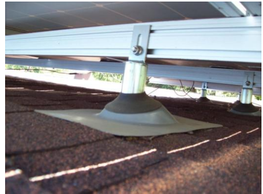
Figure 16 uninstalled flashing (incorrect)
