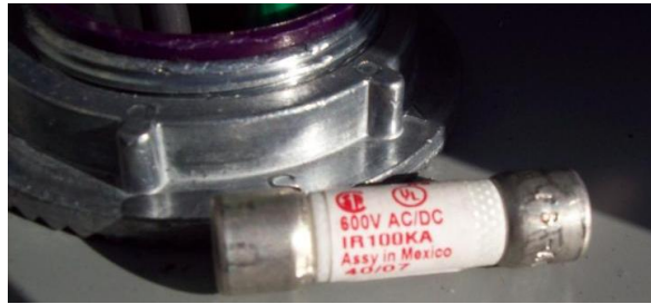
Figure 22 properly rated midget fuse (correct)
