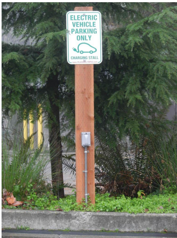
FIGURE 9: LEVEL 1 CHARGING STATION WITH SIGNAGE
