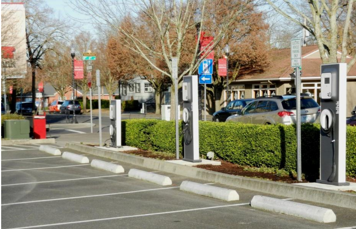
FIGURE 16: EV SUPPLY EQUIPMENT PLACED IN LANDSCAPING
