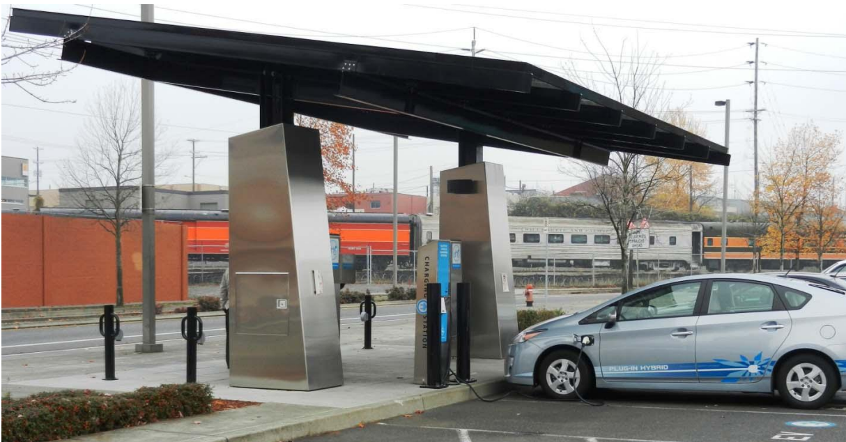
FIGURE 17: EV CHARGING STATION WITH SOLAR CANOPY
