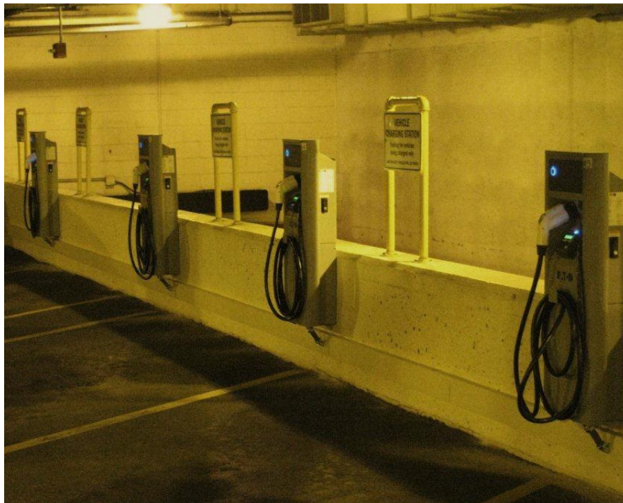
FIGURE 15: SURFACE-MOUNTED CONDUIT BELOW EV SUPPLY EQUIPMENT
