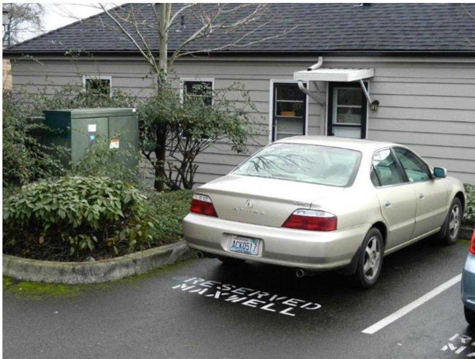
FIGURE 13: EXISTING TRANSFORMER NEAR POTENTIAL EV CHARGING STATION
