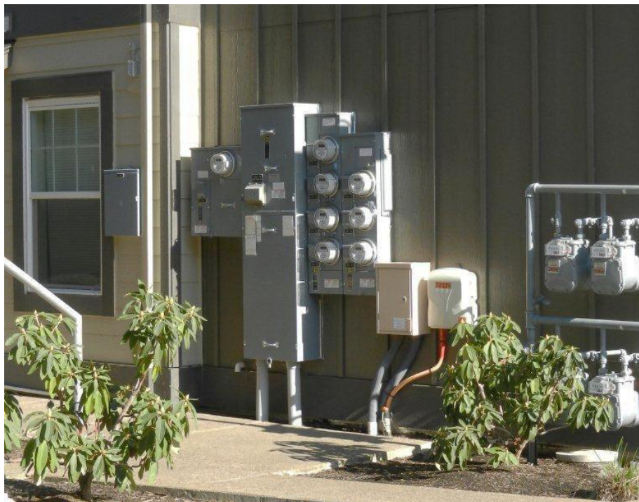
FIGURE 5: TYPICAL ARRAY OF METERS AT A MULTI-UNIT DWELLING
