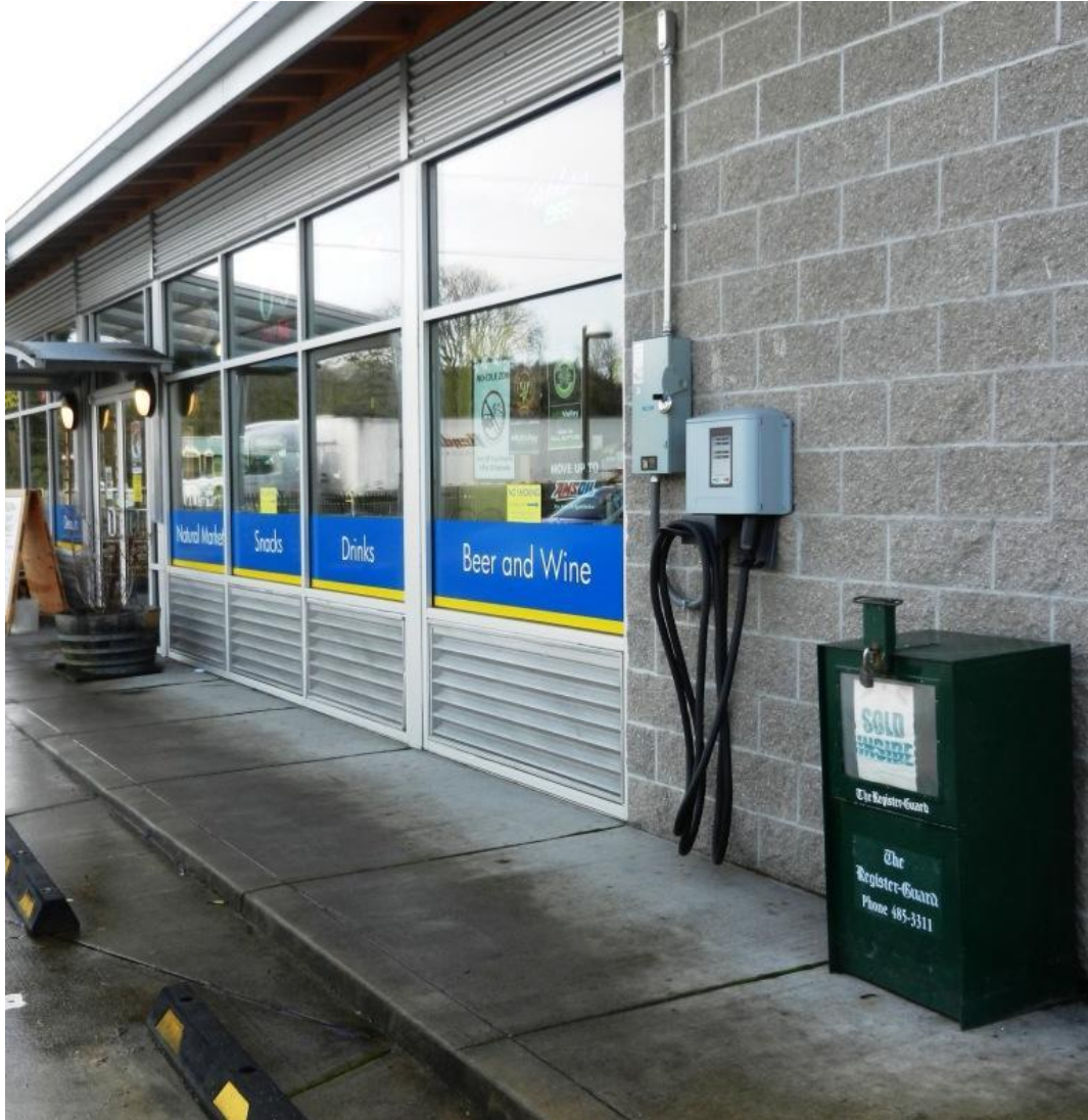
FIGURE 14: CHARGING CABLE USE WILL BLOCK SIDEWALK
