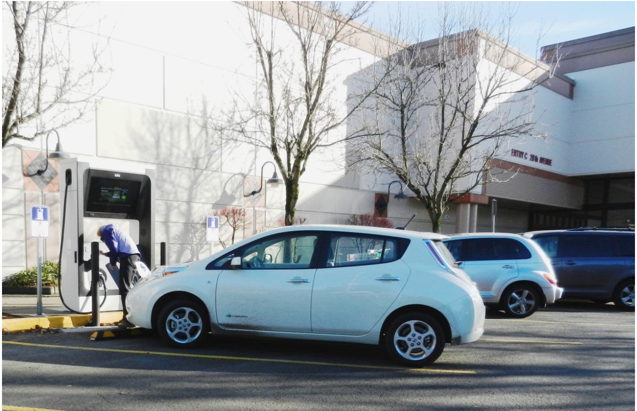
FIGURE 7: DC FAST CHARGER AT RETAIL STORE
