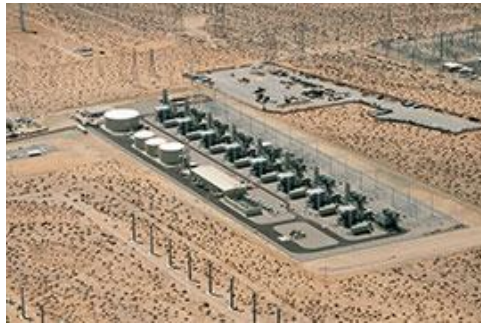
2013: 800 MW plant in California
