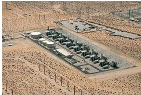
2013: 800 MW plant in California
