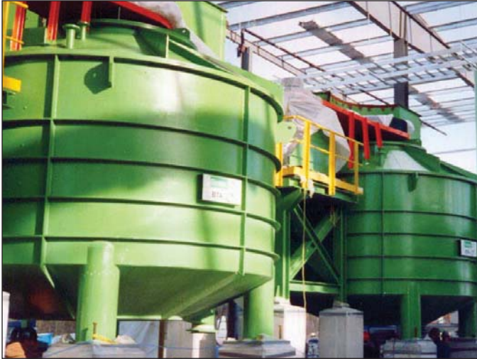
PHOTOGRAPH 1 – Pulper at Dufferin facility (City of Toronto, 2009).
