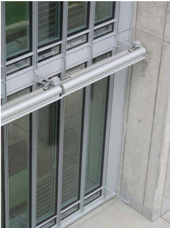
Figure 36: Detail of exterior roller shades and trickle vents
